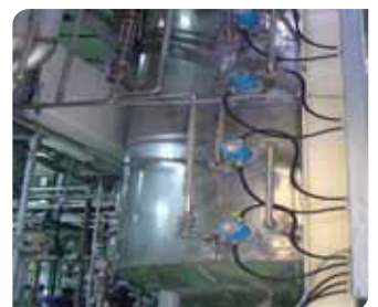
Waste Treatment System
