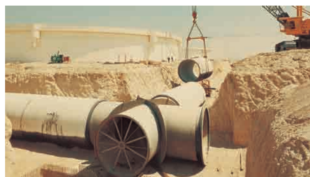
Header Tank for Main Colleting Pipeline
