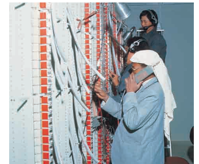
Telephone Expansion Project in Saudi Arabia • Location : Saudi Arabia • Client : Ministry of Posts, Telegraphs and Telecommunications (MOPTT) • Project Overview : 1,260,000 Circuit Automatic Telephone Installation Project - Installed Cable : 17,964m - Installed Manholes : 16,000 EA - Newly Constructed 105 telephone office buildings - Air Pump : 113 EA
