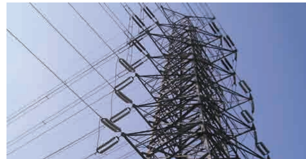
765KV Sintaebaeg Transmission Line
