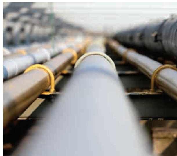
Pocheon Gas Pipe Work • Location : Pocheon, Gyeonggi-do • Client : Korea Gas Corp. • Project Overview : Gas Pipeline 30" x 46km
