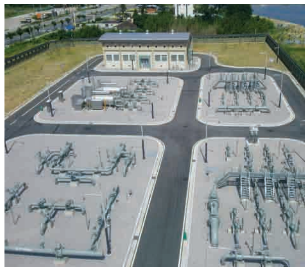
Mokpo-Haenam Gas Pipe Work • Location : Mokpo - Haenam, Jeollanam-do • Client : Korea Gas Corp. • Project Overview : Gas Pipeline 20" x 47km, 5 Control Plants
